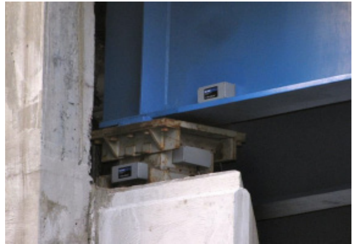
G-Link wireless accelerometer, SG Link wireless strain gauge, and DVRT linear displacement sensor monitor seismic isolation bearing.
