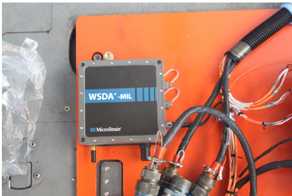
Figure 2: Wireless Sensor Data Aggregator (WSDA-MIL) installed aboard MH-60S
